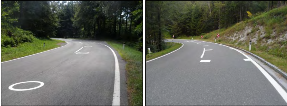
Fig. 8: Shape of road markings; A: elliptic design, B: psychological brake (bar design).
