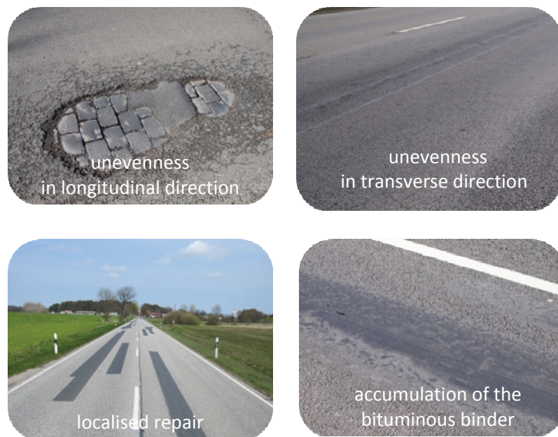
Figure 2: Examples of road surface defects
